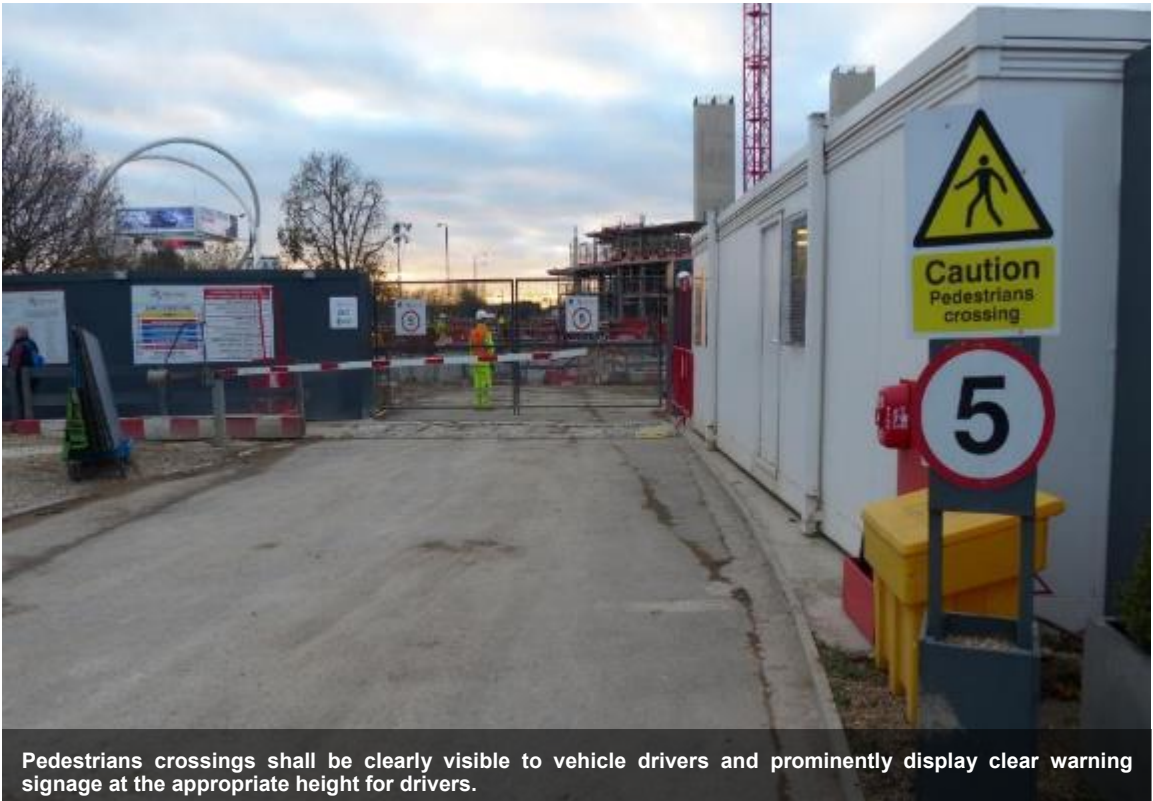
Signs shall be prominently displayed at the vehicular access points, which detail the specific rules for all drivers. A CLOCS compliance poster shall be prominently displayed at the vehicular entrance gate, so that the Banksmen or Traffic Marshals can perform the necessary checks on vehicles accessing site.
