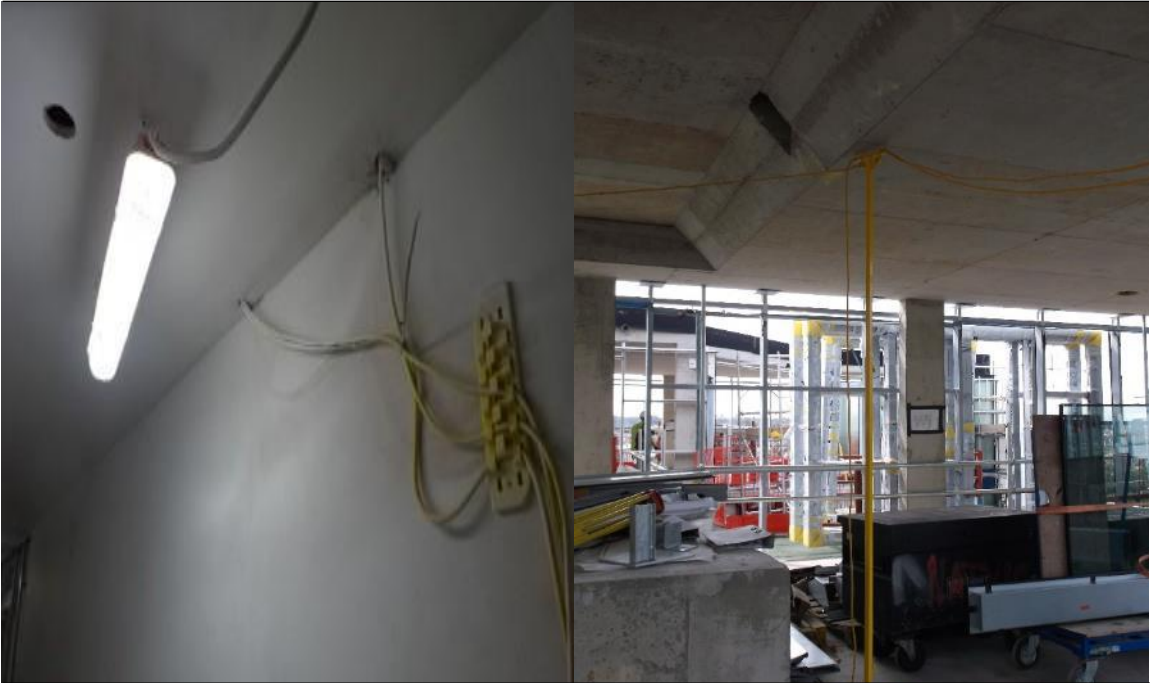
Cables and leads shall be raised above the floor level and be fixed to walls or suspended from proprietary fixings, such as skyhooks or skyhook stands. Skyhook stations shall be positioned on all floor levels.
