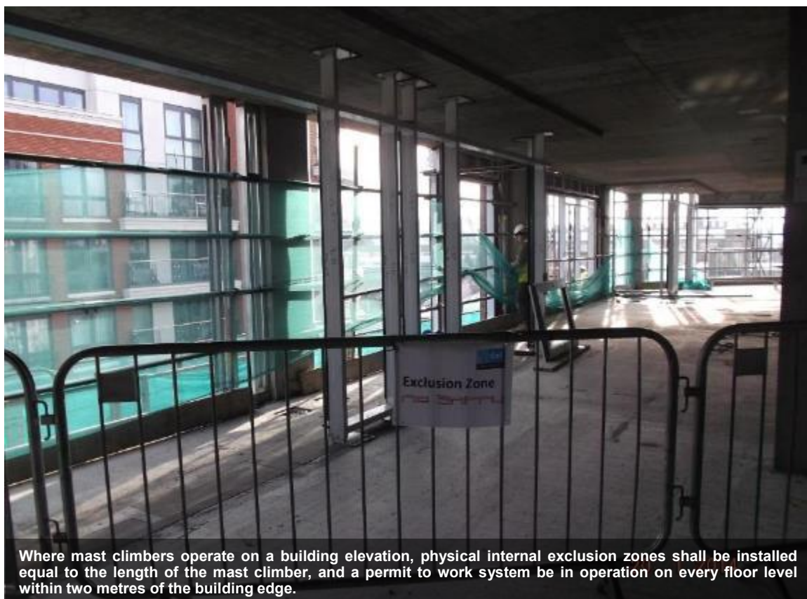
Mast climbers shall be located within a physical exclusion zone, have debris netting wrapped and secured on all sides and below, and be subject to a permit to work system.
