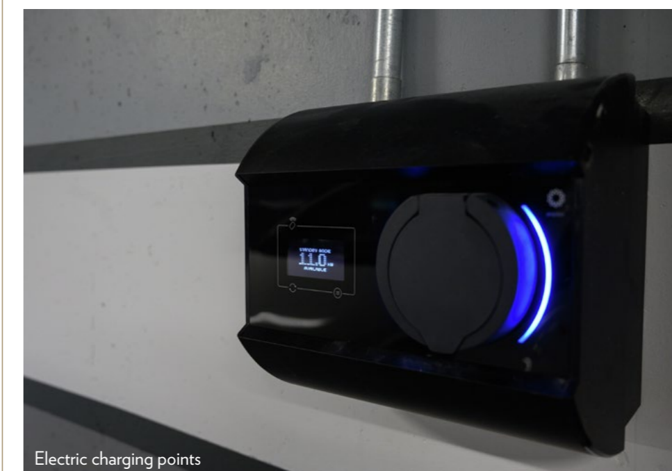
Electric charging points
